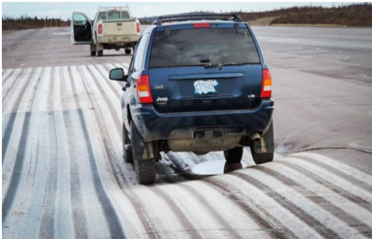
Figure 6. Dip in the Inuvik Airport runway caused by permafrost thaw. Source GNWT.
